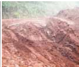
Sight of the bad patch as seen next morning
